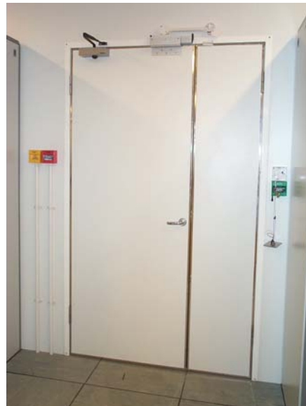
Door and a half with magnetic lock
