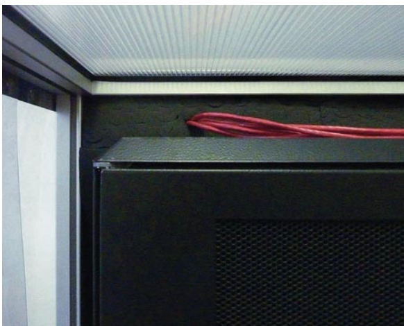
Cable openings at the bottom of the cabinet are sealed airtight with the CoolControl Xpand.
